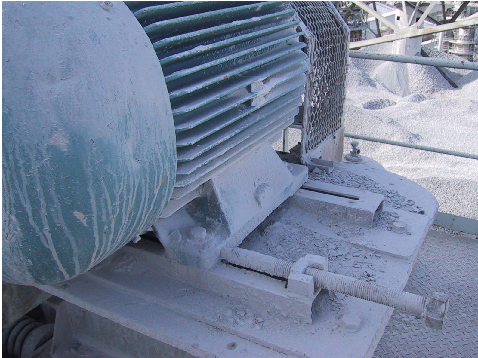
CORRODED TENSION RULERS
